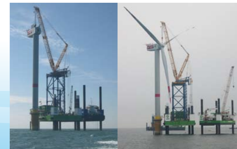
Superlift backstay wires allow the crane to lift the 320 tons nacelle at a reach of 22 m while using only 150 tons counterweight
